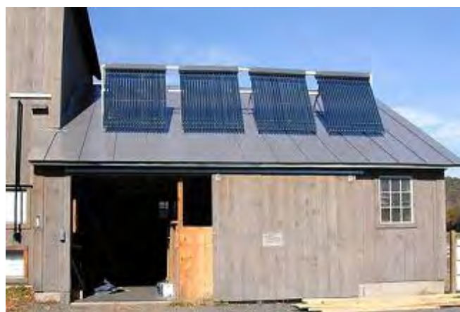
EXHIBIT 4-28: Evacuated Tube Solar Water Heating System on a Barn in Massachusetts
