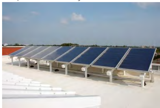
Flat panel collector system
