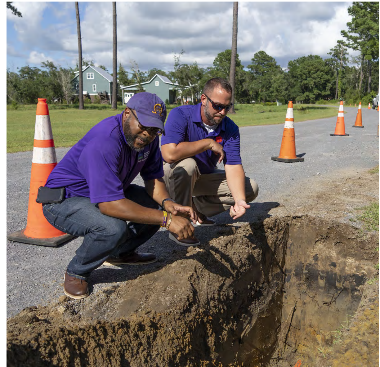
Home Telephone Company, Inc employees perform directional drilling to insert underground fiberoptic cables, part of the U.S. Department of Agriculture USDA Rural Development RD ReConnect 50/50 grant.
